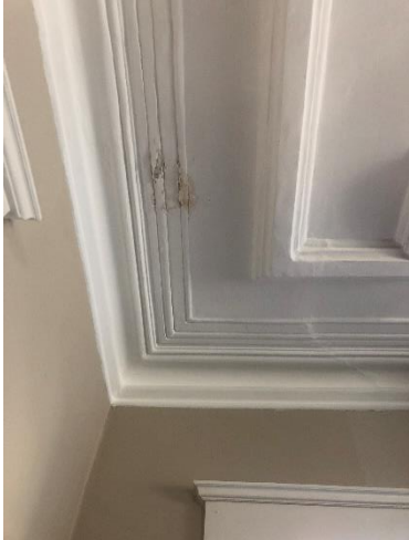
Fig. 49. Photograph by Claire Buchinger. Living Room Water Damage, Facing West . April 2, 2023. Ithaca, New York.
