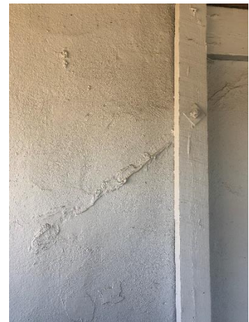
Fig. 41. Photograph by Claire Buchinger. Exterior Stucco Patching . April 2, 2023. Ithaca, New York.
