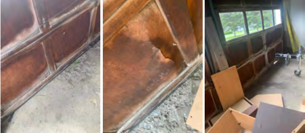
7. Detached Garage Door Operation: Manual - Loose or missing hardware, improve function
