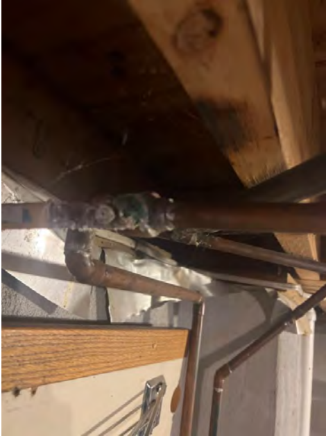
Laundry Sink Basement
