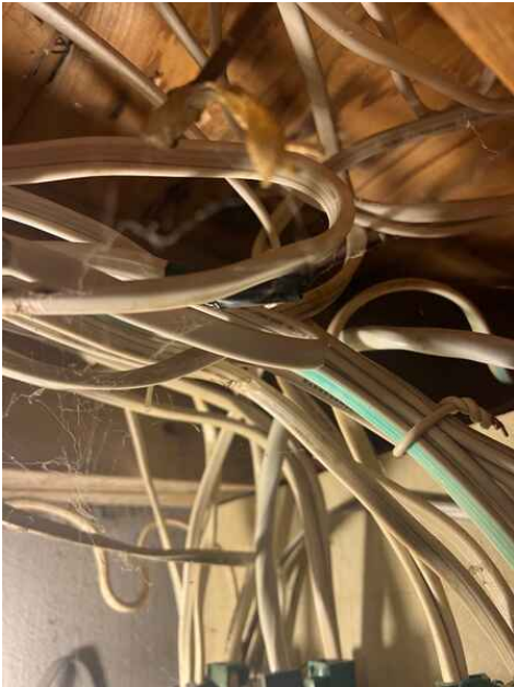
Above Electric Panel
